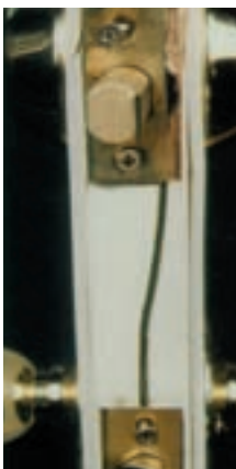
A wood edge steel door cracks under force of one hit of a 100lb. test weight.
